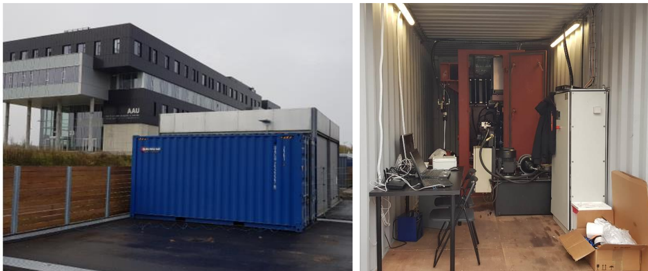
Figure 3. Floating Power Plants small-scale PTO dry-test rig at Aalborg University.
