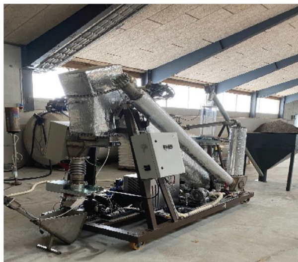
The finish plant installed in Nibe - Denmark
