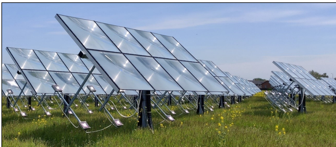
Fig.1 Photo of the Fresnel lens solar collector field, Lendemarke, Denmark.
