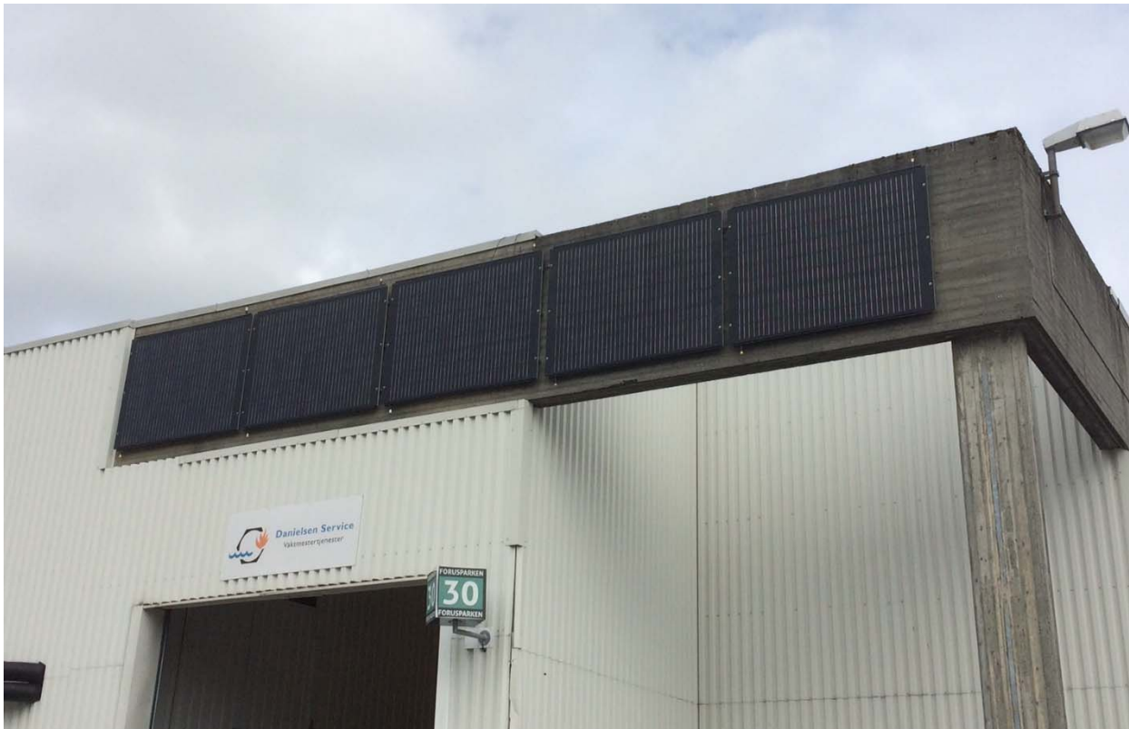
Figure 4.2(B).6 Large PVTE modules fixed to the concrete façade by drilling through the modules
