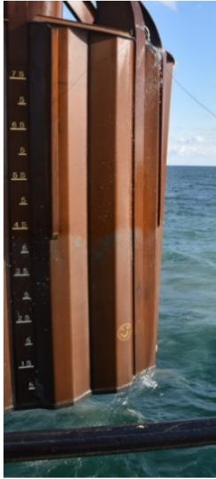
Figure 3. Observed skirt deflection.
