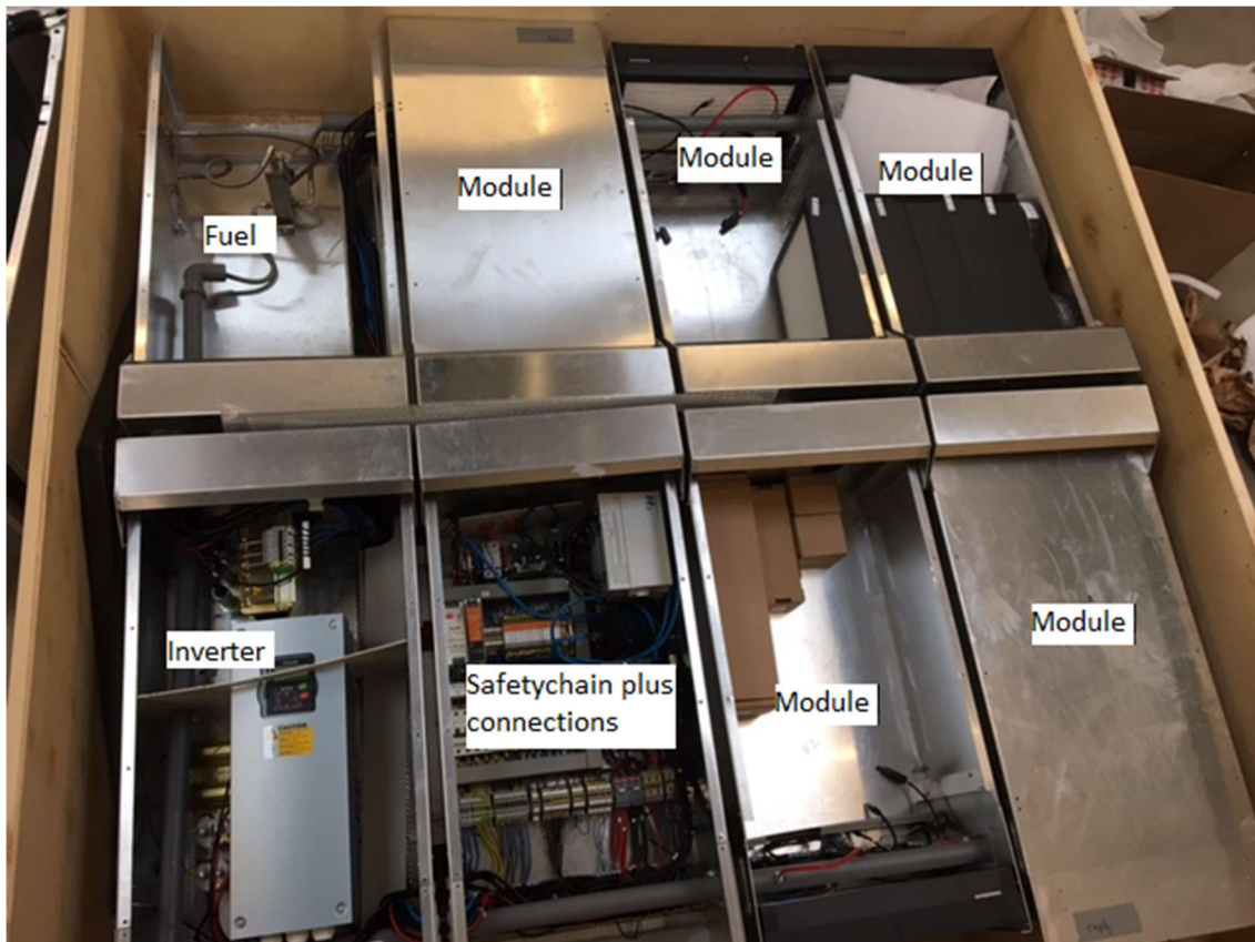
Figure 21: Assembled roof top box, excluding fuel cell modules and fuel feed system.
