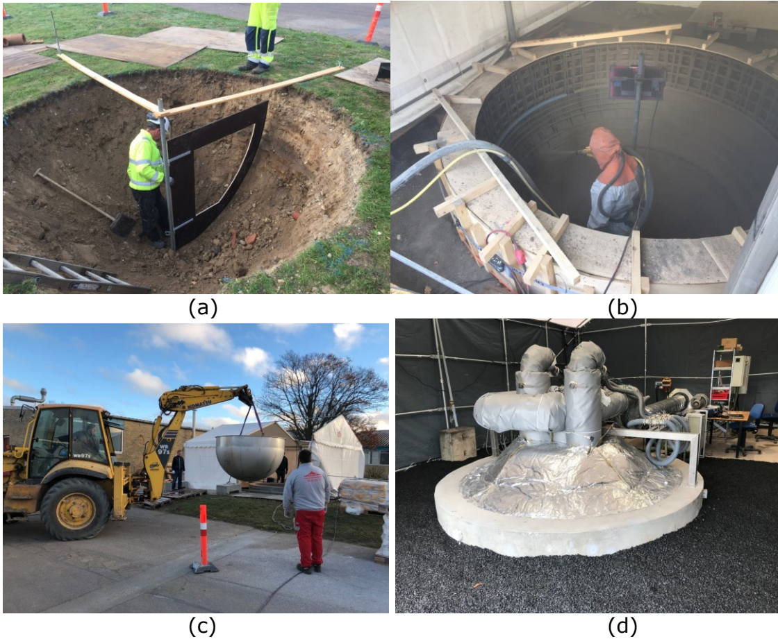
Figure 5. Construction of the vertical flow rock bed storage: (a) excavation, (b) spraying concrete onto the steel support frame, (c) installing the stainless-steel shell, and (d) final assembly with heaters, fans and insulation installed.
