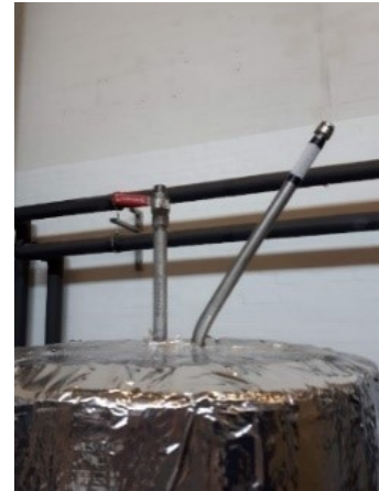
Fig. 7. Two pipes in the top of the PCM storage.
