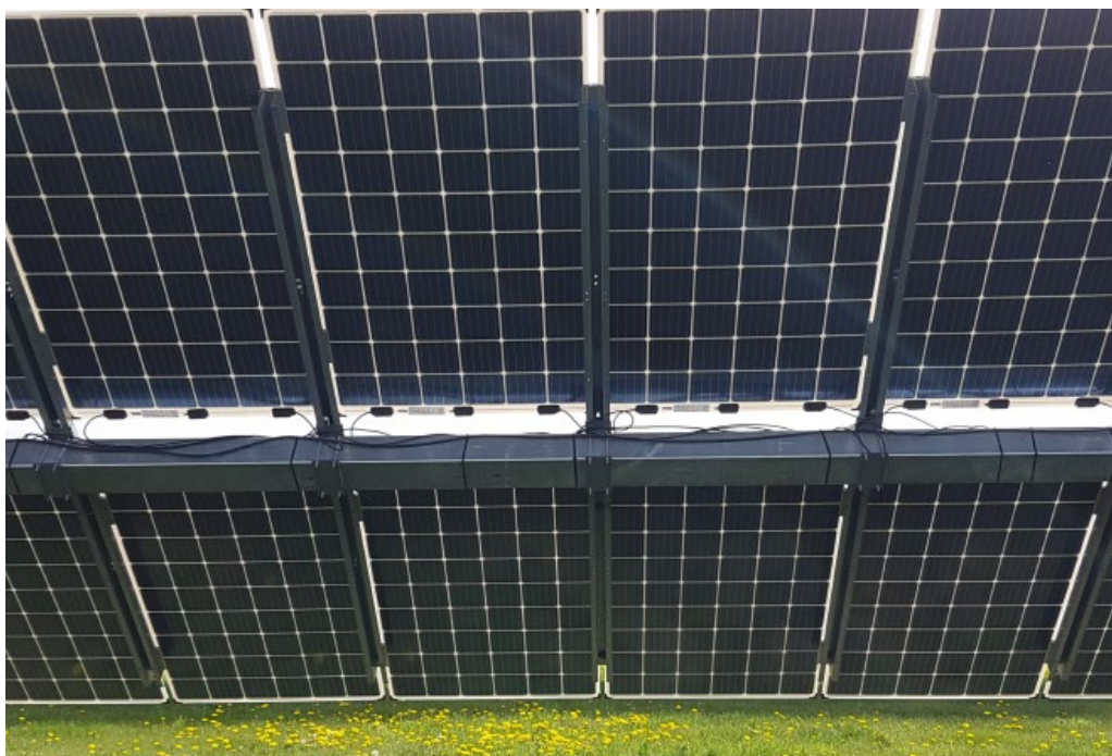
Figure 3 – backside view of bifacial PV panels.
