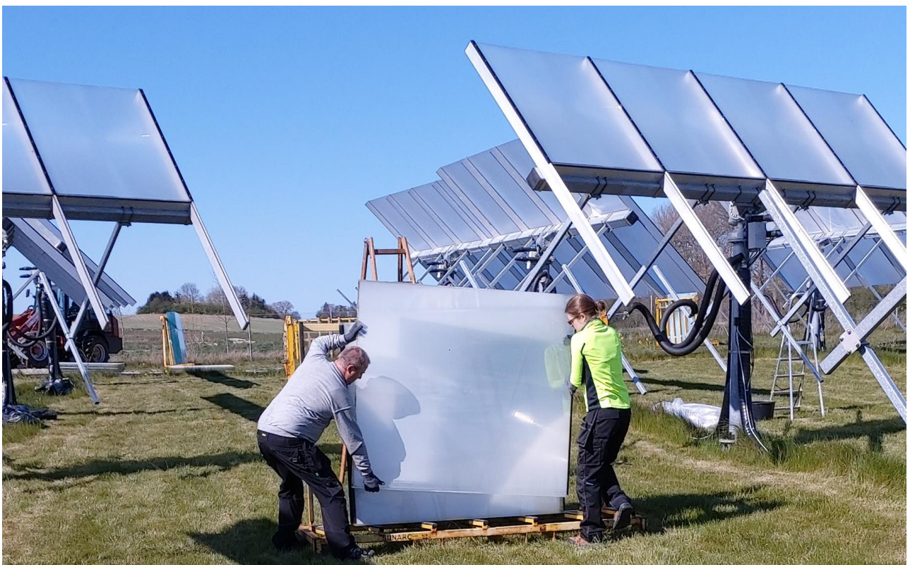
Silicone lens installation on Lendemarke. The lenses are opaque due to the casting film still being on the lens to prevent uncontrolled focal points during installation.
