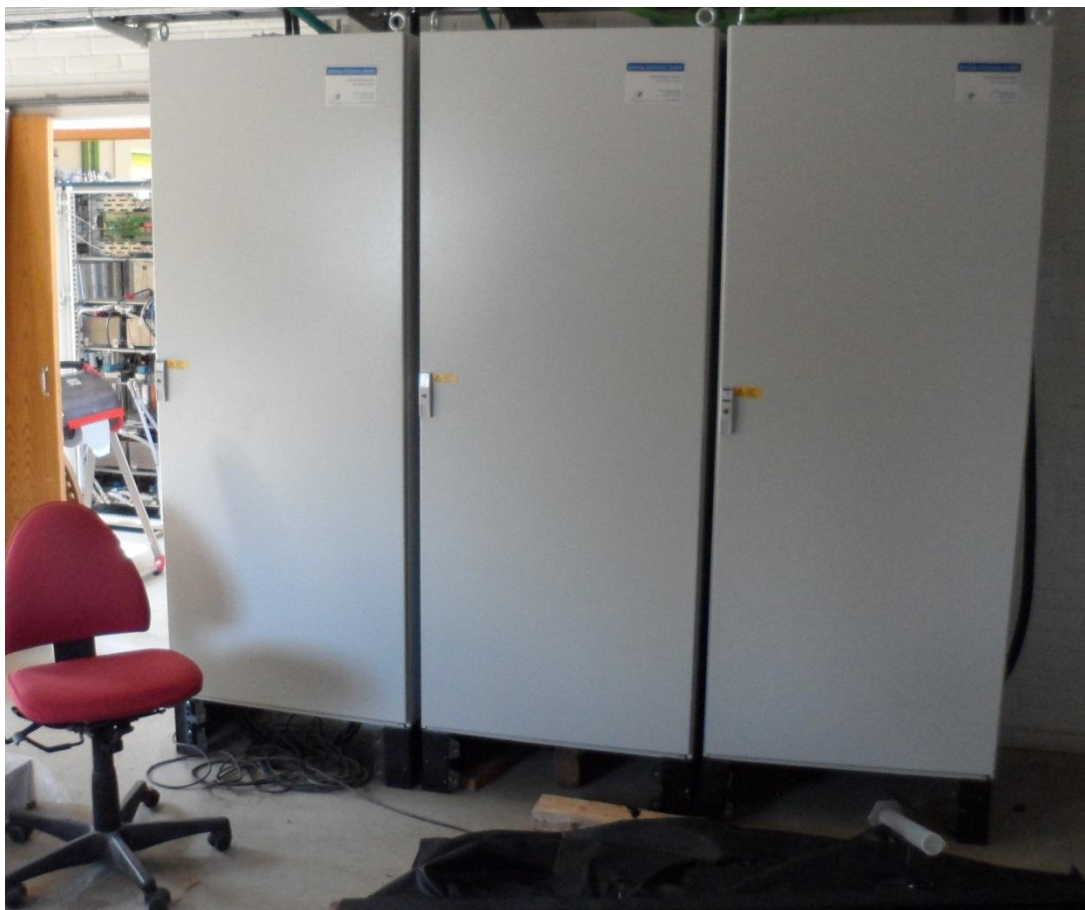
Figure 6: Each of these three ac/dc converters is able to deliver up to 600A DC for the electrolysis stack. The H2Cost-2 project required addition of the third converter in order to operate the stack at 600 mA/cm 2 .
