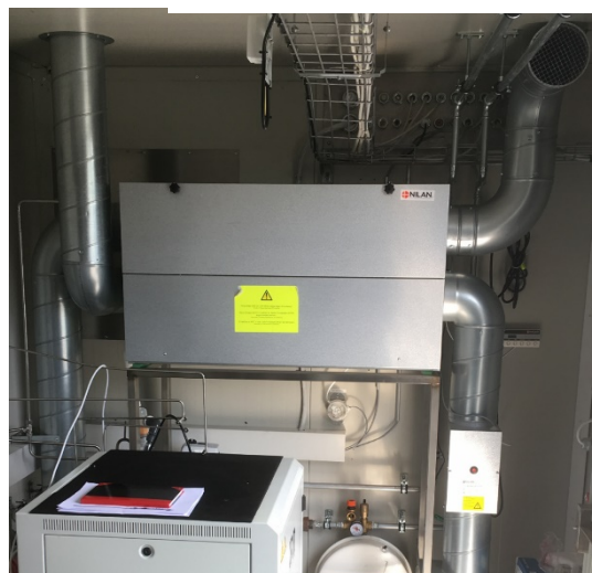
Figure 4. Ventilation system with heat exchanger installed in the 20-ft container.
