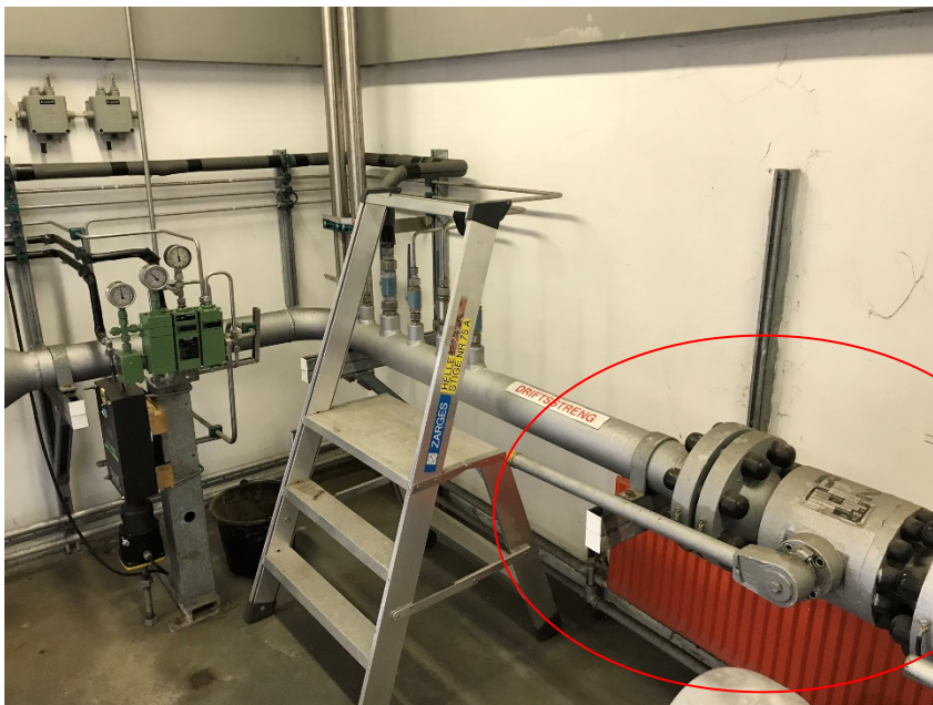
Figure 24. Picture of the leaking valve in M/R Helle.
