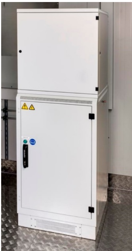
Figure 5. PEM electrolyser with drying system on top.
