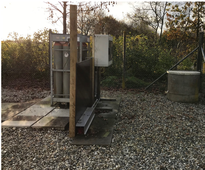
Figure 11. Picture of the hydrogen storage.
