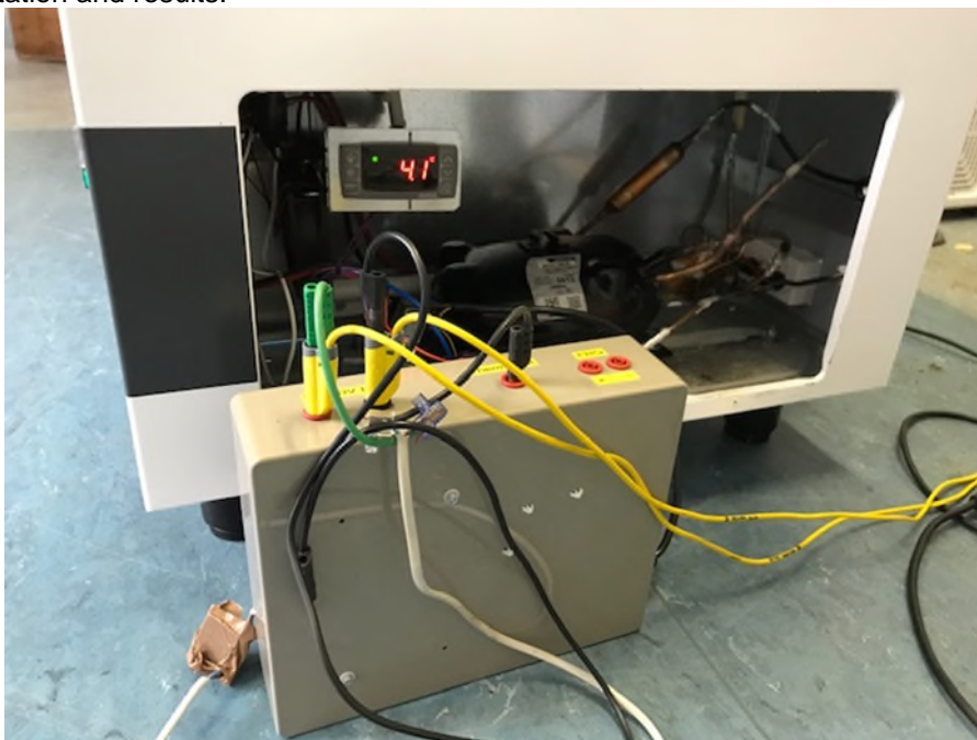
Figure 54 Compressor with external power supply
