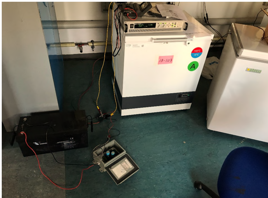
Figure 39 Charge regulator and battery connected. The PV simulator is seen on top of the refrigerator cabinet.
