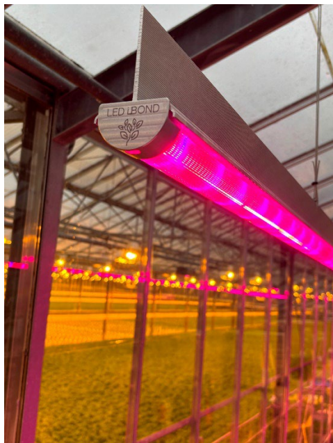
Figure 28: 9m single line Hortisaber in LEGRO's test area - easily provides the necessary light level
