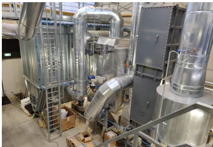
Tight emission thresholds in the NL require extensive flue gas cleaning at small scale district heating CHP plant: 2 x SNCR + cyclone + SCR + economiser + bag filter + condenser. Photo by ProBiomass BV.
