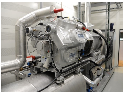
Figure 6: One of the installed 500 kW heat pumps.
