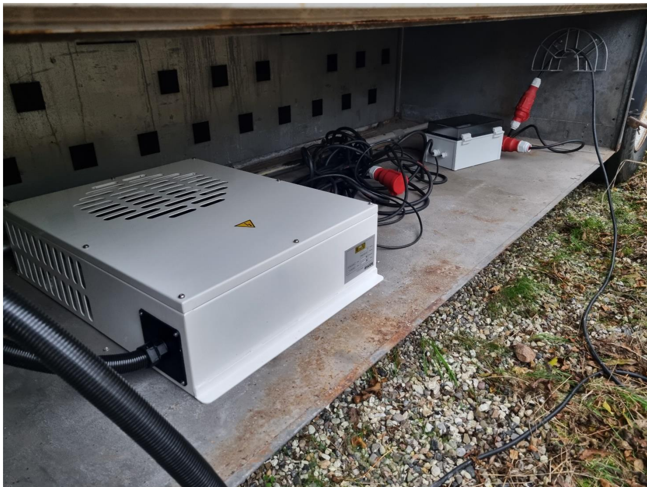
Charger mounted in pallet box, of the trailer.
