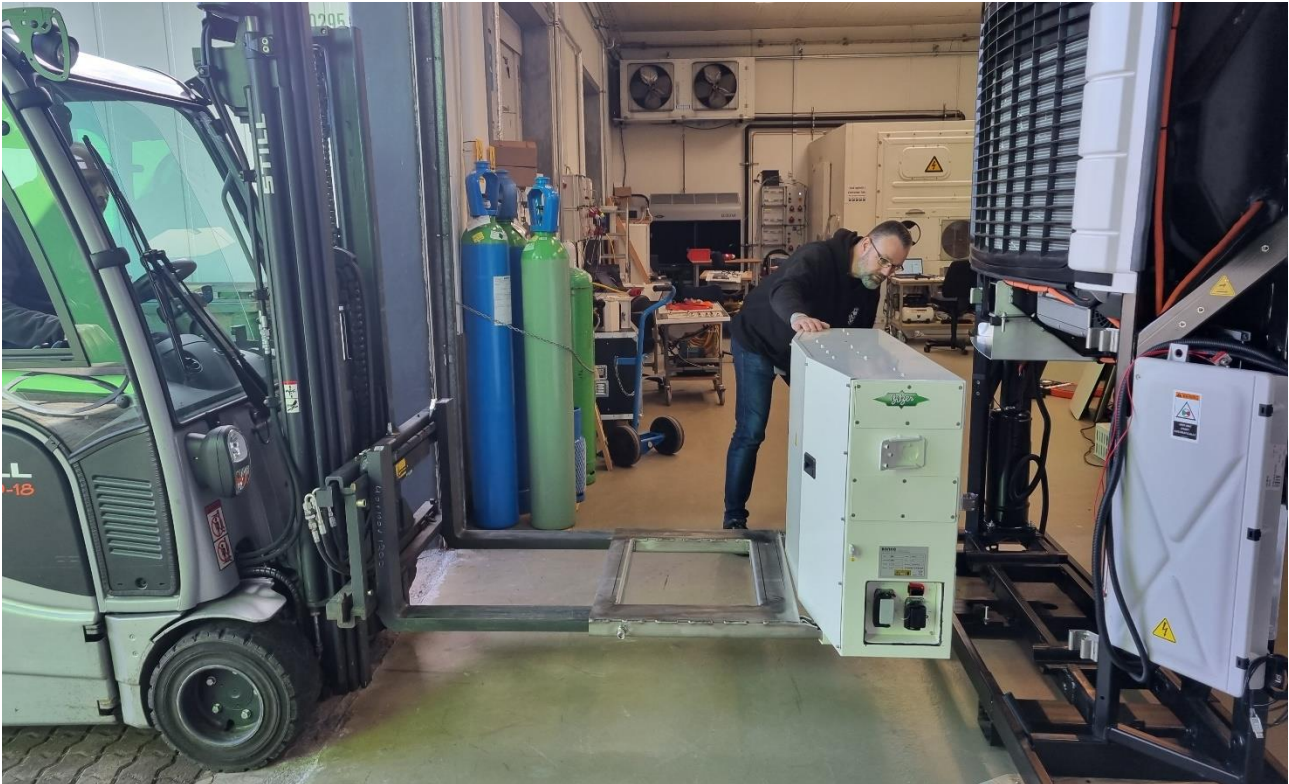
Battery being installed using forklift adaptor. Changing a faulty battery can be done in 30 minutes if needed.
