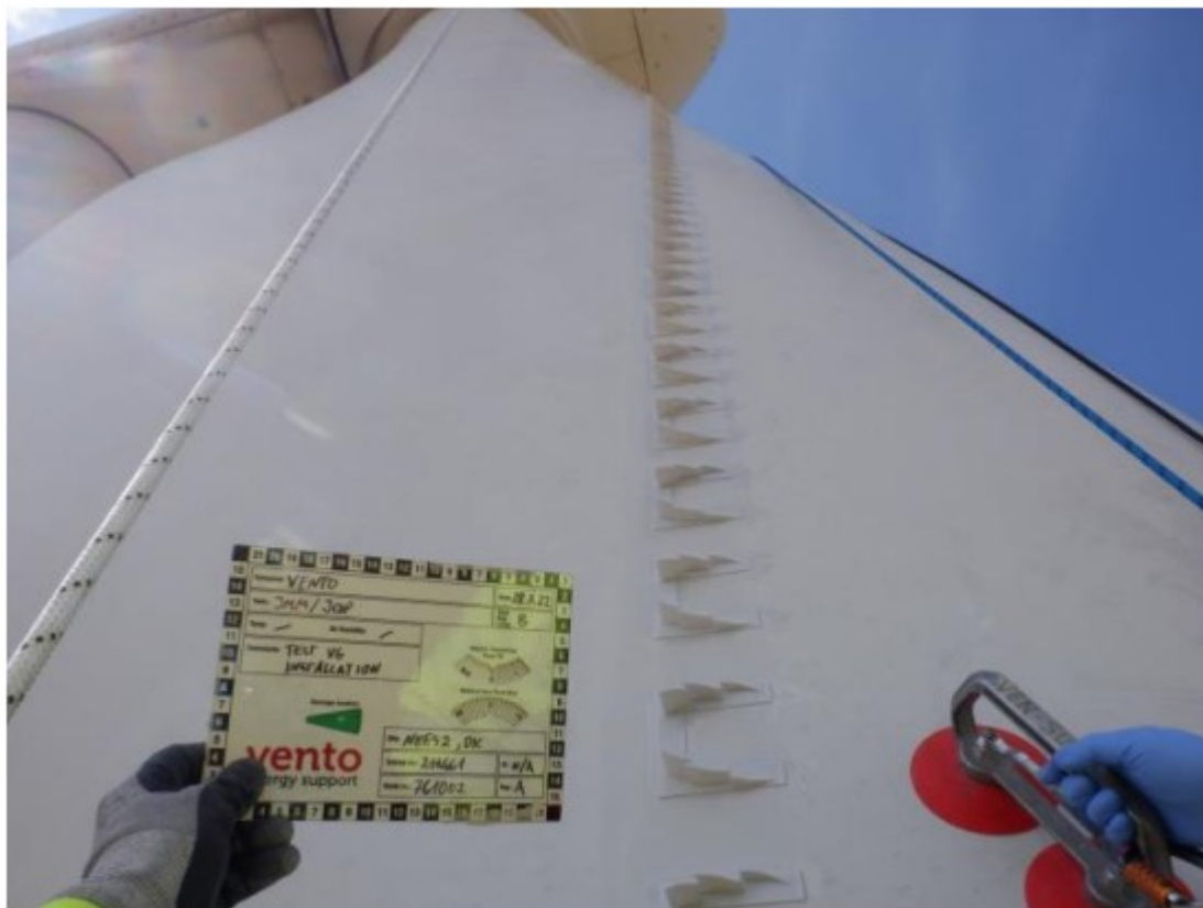
Figure 10: Installation of the AdvancedVG glued to blade by double adhesive tape and sealed at the edges to prevent water to enter the adhesive area.
