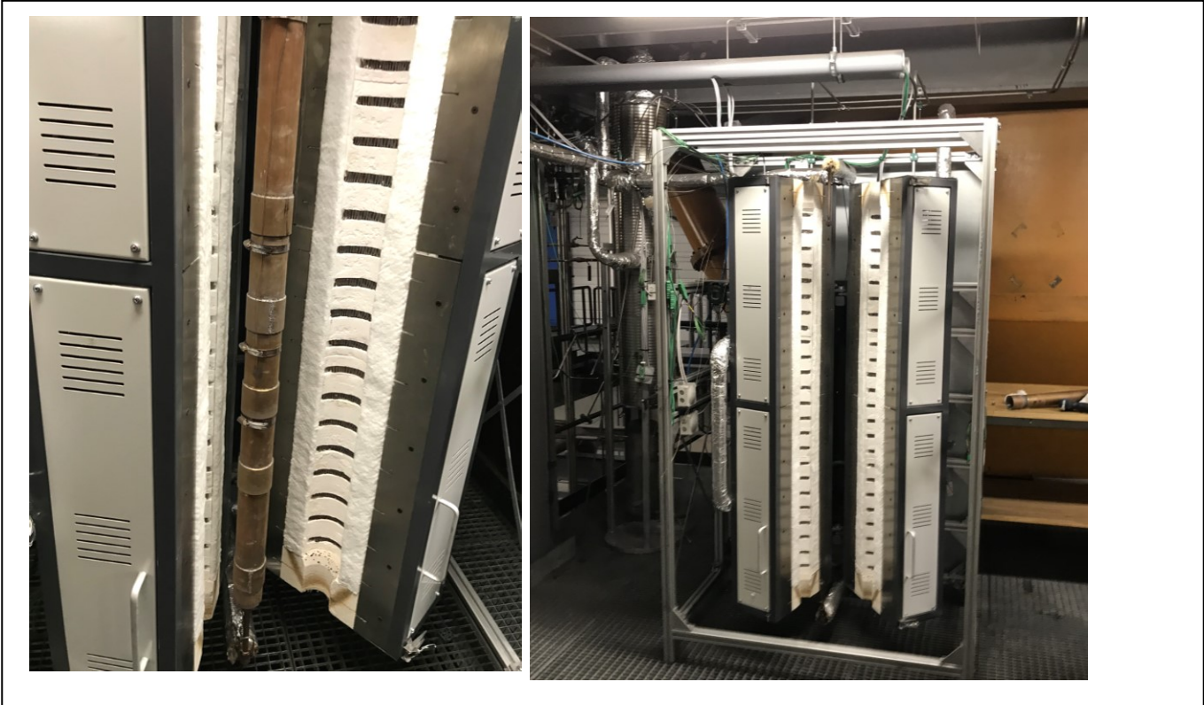
Figure 8. Pictures of the setup used at Skive Fjernvarme
