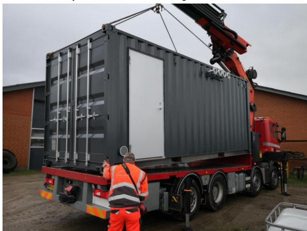
Loading of Nature Energy Midtfyn heat pump
