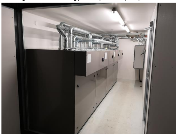
Heat pump ready for delivery
