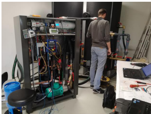
Test and logging performance results early state of heat pump. Test facilities has been rebuilt multiple times to fulfil shifting needs and optimize stability.
