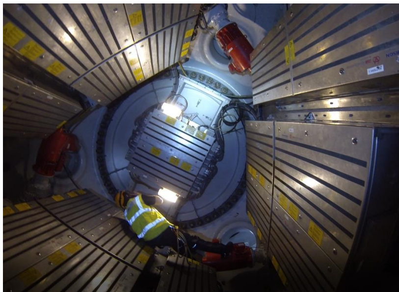
Figure 28 – Technician inspecting cabling inside hub of LDT
