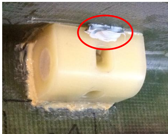
Figure 89 – Photo showing the 60 to 80-degree bracket installed in the PS/TE corner, being held in position by very fast curing SikaForce 7800 BLUE while primary adhesive is curing
