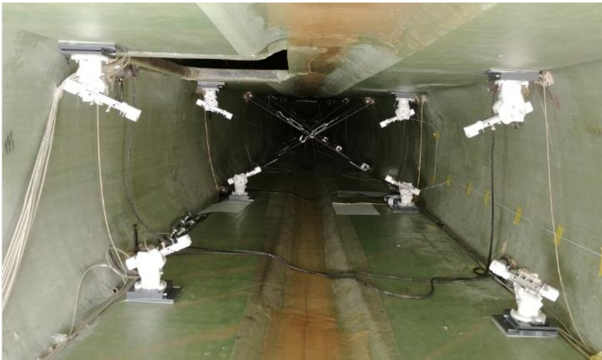
Figure 76 - CSSDS test integration at DTU, installed FCMs inside the blade (left) and test rig (right)
