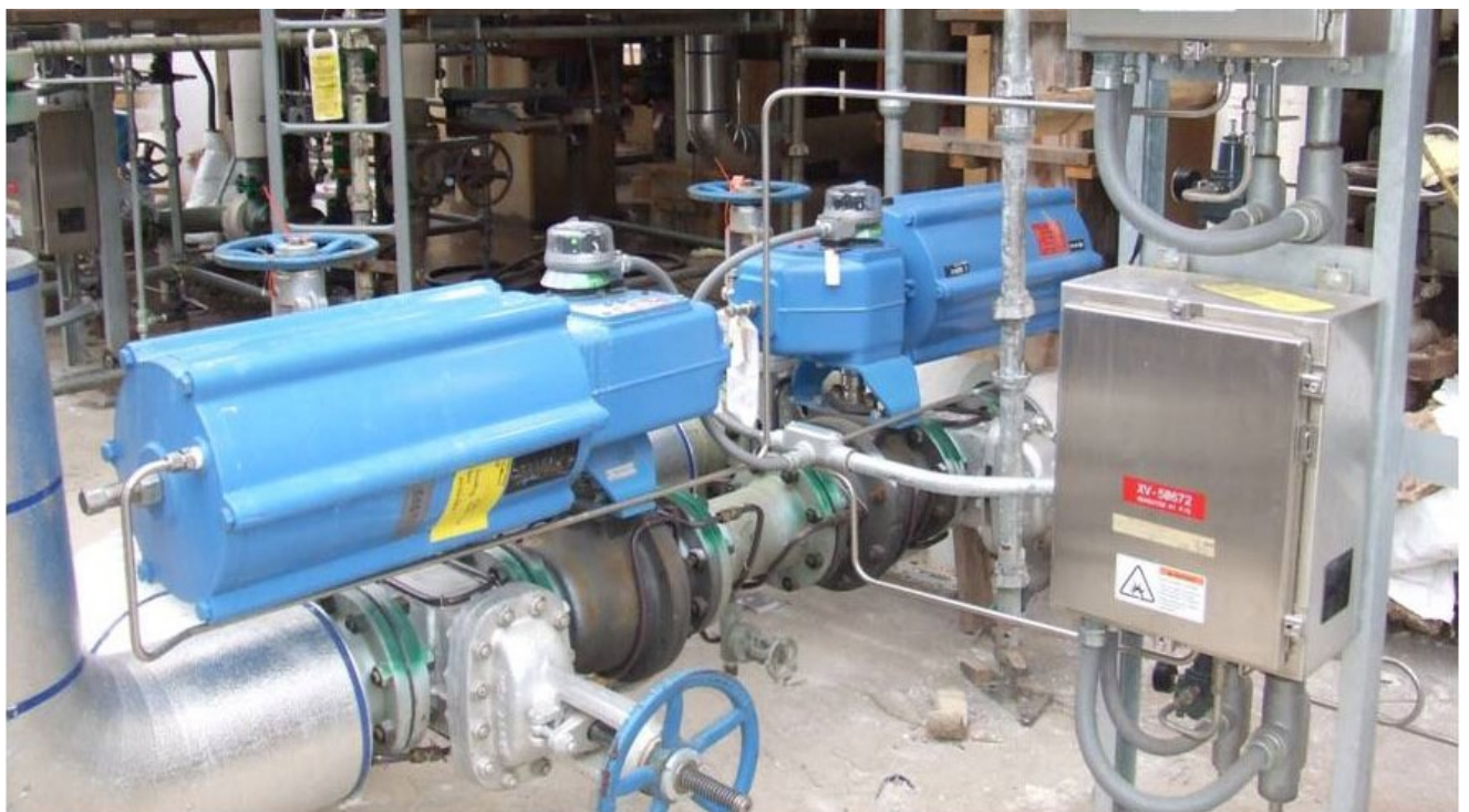
Picture 3.3: Gas train with low pressure drop and ball valve.
