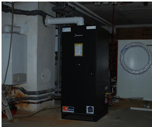
Installation: Kellberg VVS
