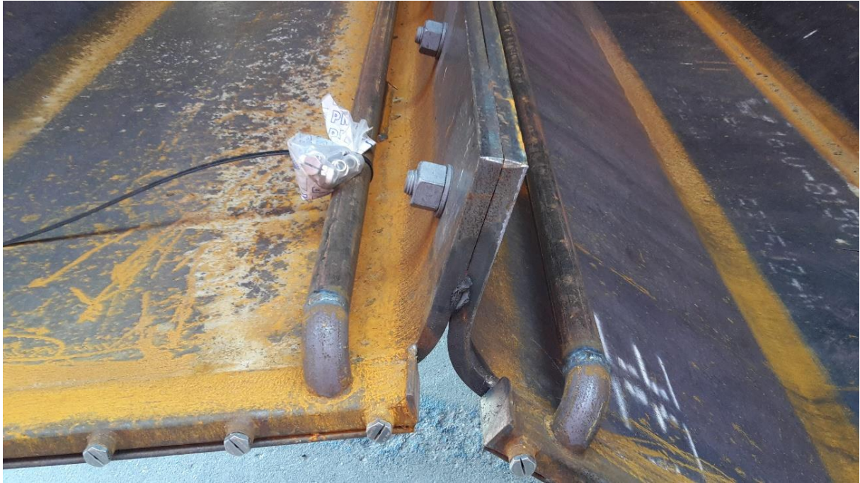
Figure 22 Flushing pipes and panels
