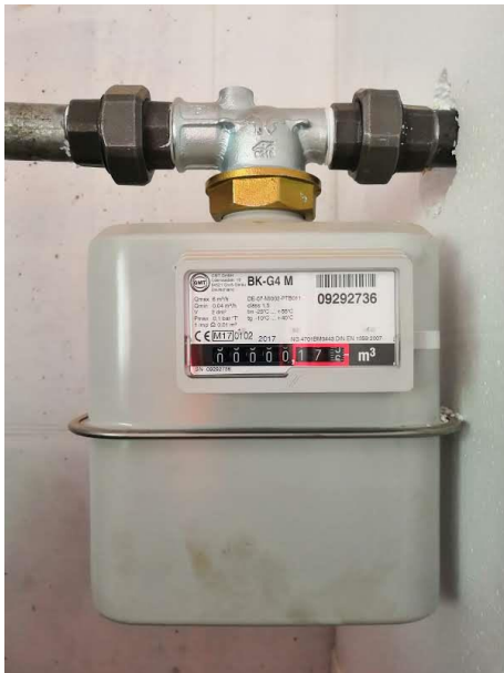
Figure 25: Gas meter mounted on the pipe at from the digestion chamber
