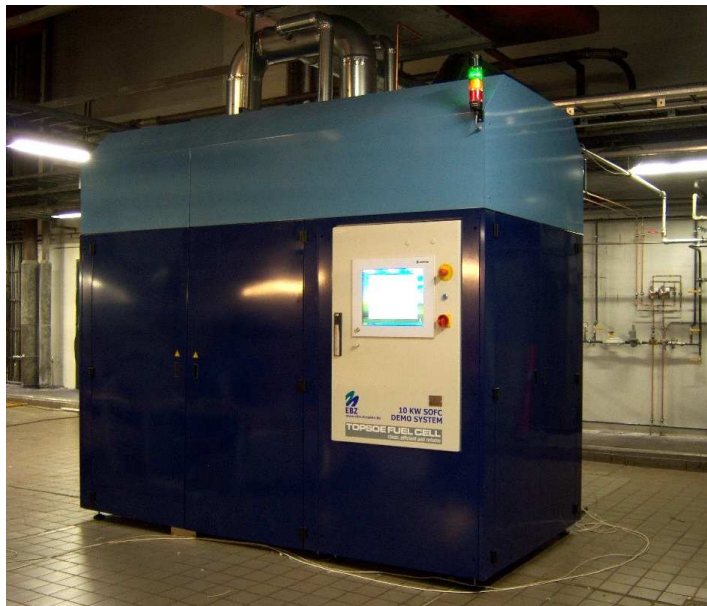
Figure 2: The 10 kW SOFC demonstration unit in place at H.C. Ørstedværket.
