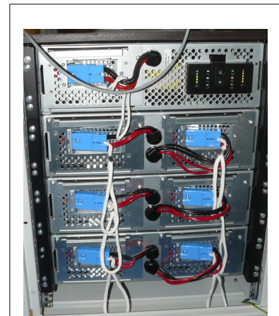
Illustration 13: UPS and battery packs
