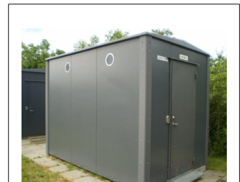
Illustration 1: POP station in Kolding prior to installing vandal proofing of the intake / exhaust
