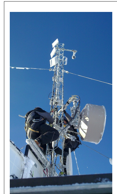
Illustration 26: Norwegian technicians servicing a telecommunication tower on a mountain peak 1600m above sea level
