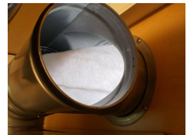
Illustration 18: Intake filter closeup
