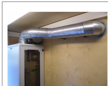
Illustration 17: Exhaust and intake ducts
