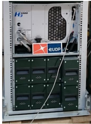
Figure 8. Power system. The battery system is placed in the bottom of the rack (offers 10 kW@15 minutes, 20 kW@6 minutes).
