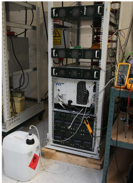
Figure 7. The UPS power system with integrated fuel cell module. The Methanol fuel tank is placed at the floor.
