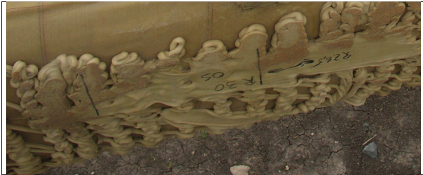
Figure 13: Insufficient bonding material found between the load carrying box and blade shell.
