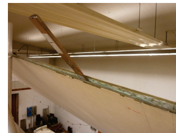
Figure 5. Blade damage in the trailing edge, with the chisel used to introduce the damage
