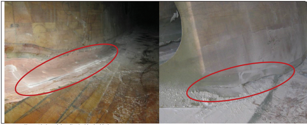
Figure 12: Spar debonding inside the blade
