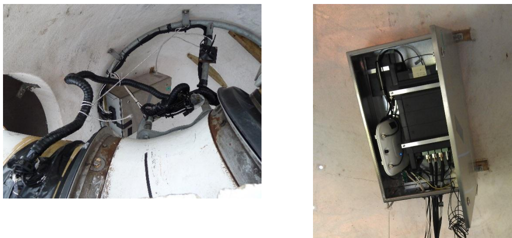
Figure 6. B&K data acquisition unit inside a waterproof box, mounted inside the spinner of V27 wind turbine. The unit accompanied by Cisco access point for wireless data transfer to the nacelle.
