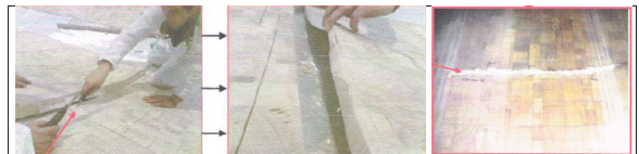
Figure 11: Transversal cut in glass layers that might lead to transversal crack in blades
