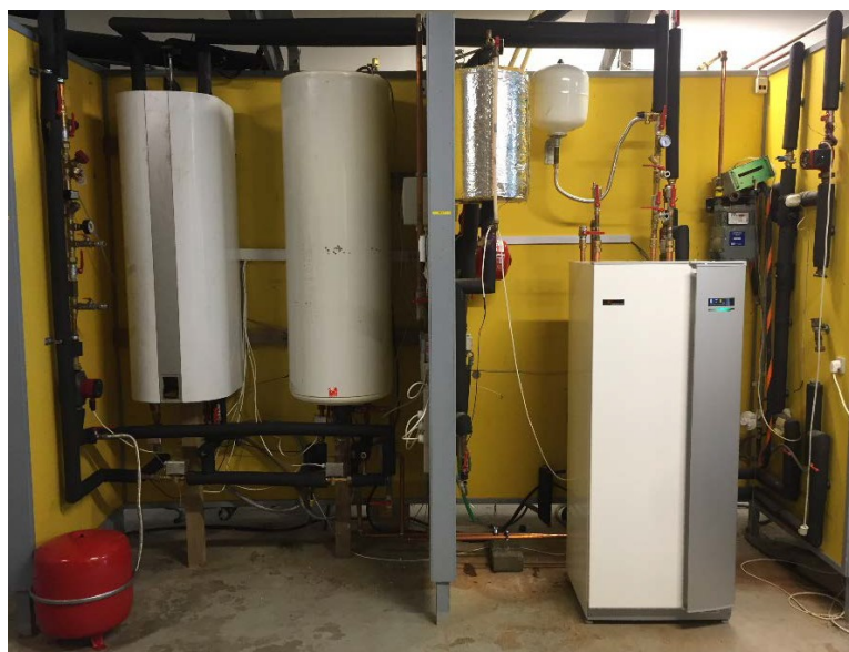
Figur 9. Indoor installation of two storage tanks and a liquid/water heat pump.
