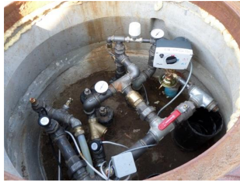
Figure 1-3 Mixing shunt placed in the demonstration area, mixing the supply temperature to supply 40°C.
