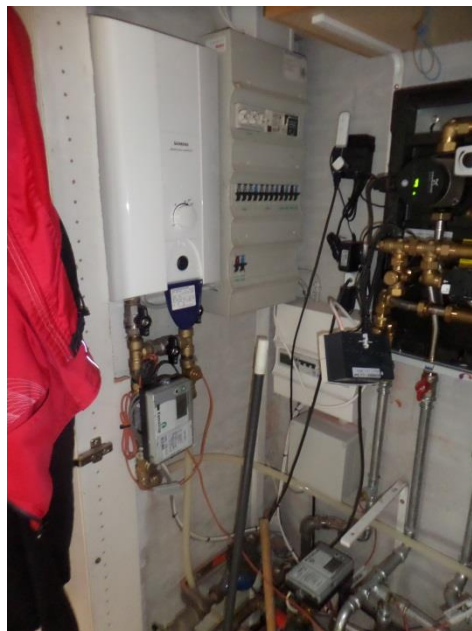
Figure 1-7 In-house installation of unit system with electrical booster and data acquisition system
