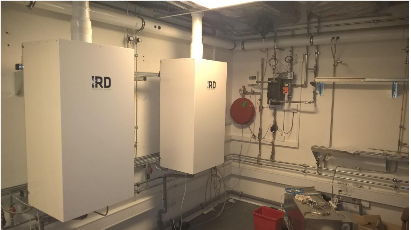
Fig. 10 Work-/test-room at TREFOR premises with installation for simultaneous test of in total four (4) \mu CHPs.
