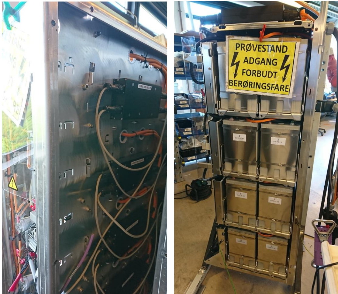
Figure 7: Battery pack for garbage truck with hot swap battery modules developed by Banke. Left side: BMS from Lithium Balance installed on the battery pack, Right side: battery modules that are hot swap enabled.
