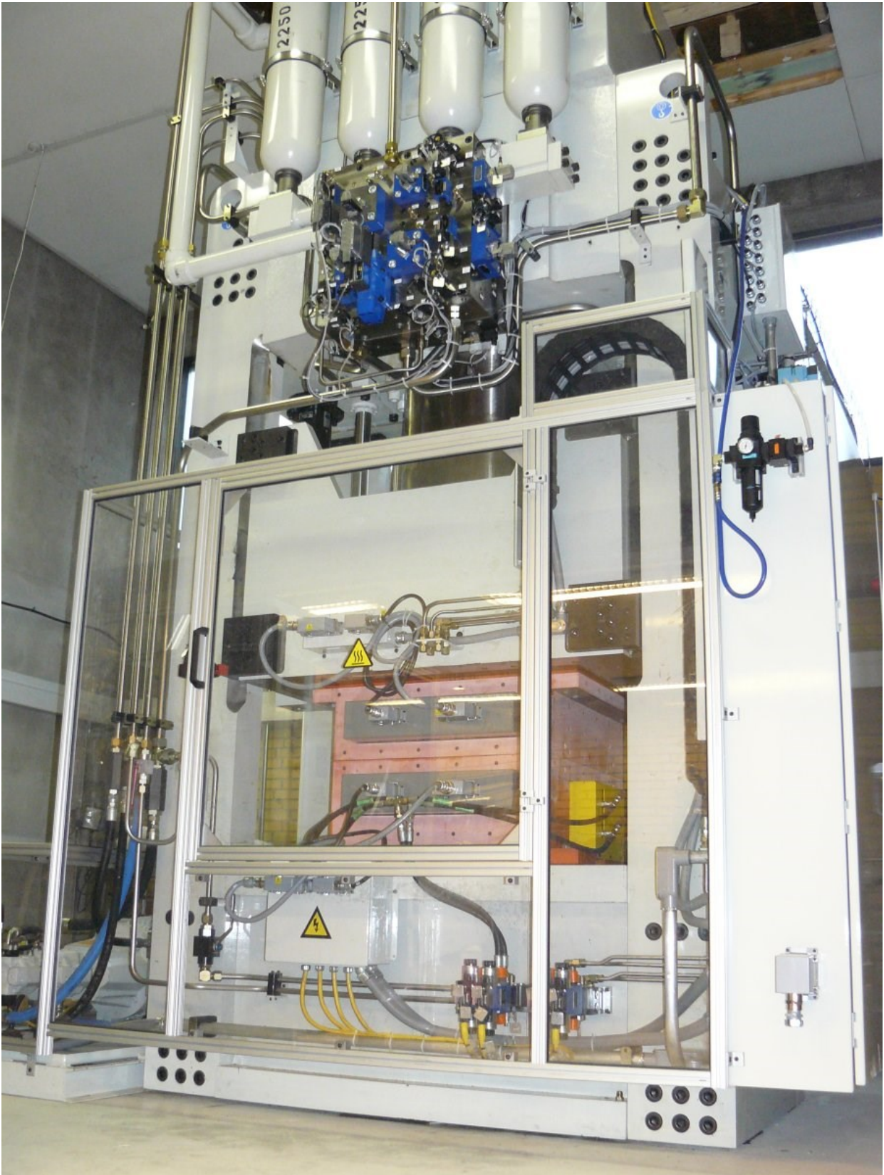
Figure 1.3.b: The 700 tons hydraulic press with the molds for hot pressing flow plates.
