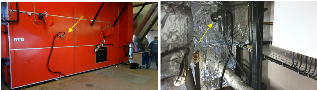
Figure 6. Left: NIR camera installed in the right side of the Hinnerup boiler. Right: RGB camera installed at the end of the boiler.
