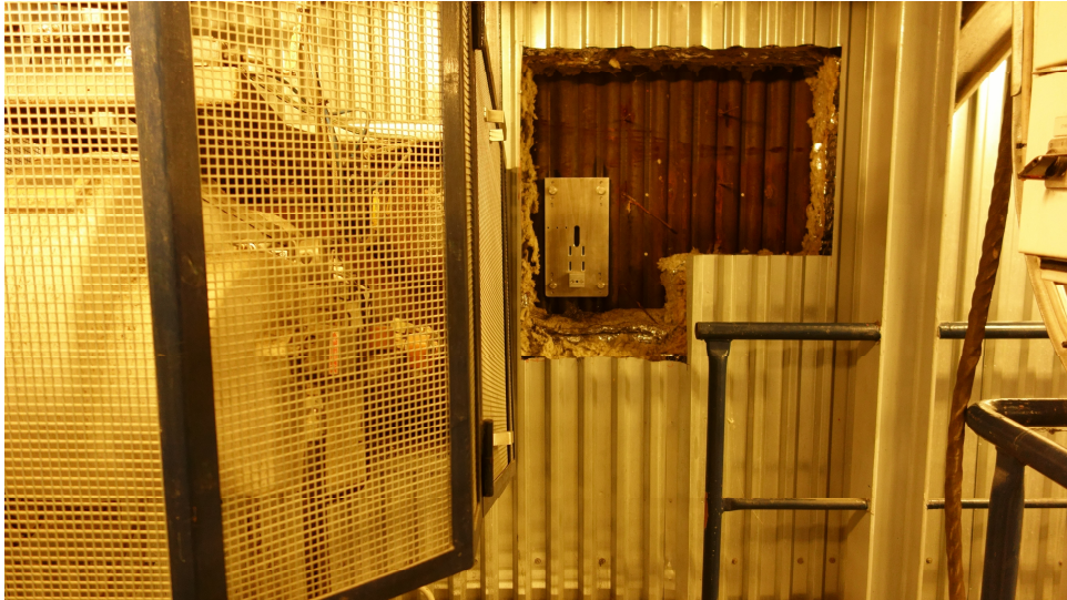
Figure 23. Mounting flange mounted on the boiler wall.
