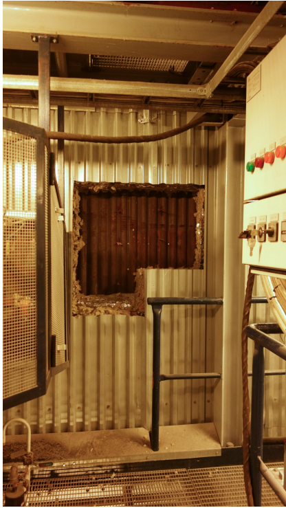
Figure 22. Preparing installation of camera. Cut-out (incorrectly too large) of insulation and cover to the right of the start-up burner.
