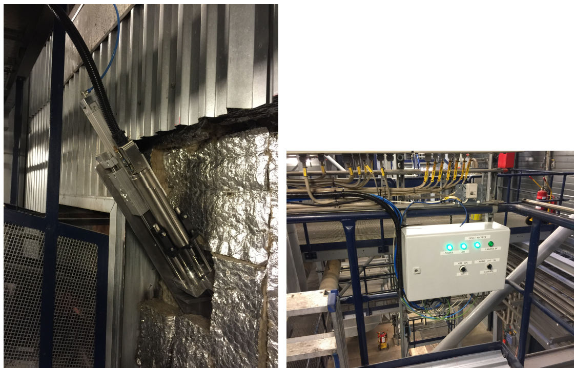
Figure 27. Left: Camera (in steel cylinder) mounted in extraction system mounted on the boiler wall at MSK. Right: Control/interface box mounted close to the camera. The black hose contains connections between the camera and the control/interface box. The blue hose is supplying compressed air for the extraction system.
