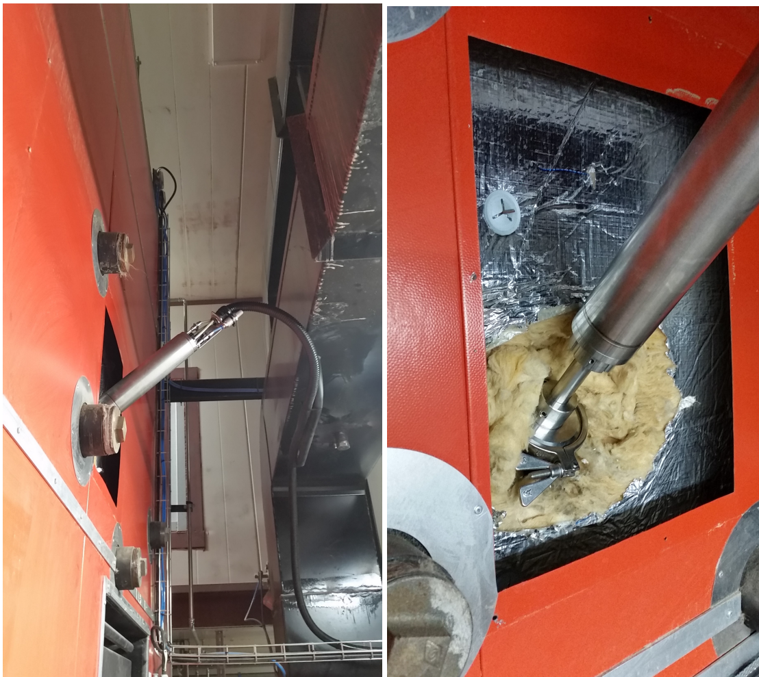
Figure 17. Left: Camera housing mounted in the middle guide tube of pellet boiler of Halsnæs Forsyning. Right: Camera flange and camera housing.
