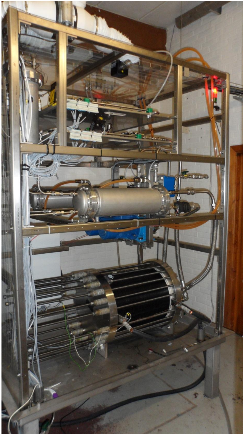
Figure 20. Bare minimum electrolyzer system build in the HyProvide for testing purposes.
