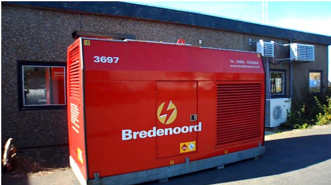
Figure 23. Diesel generator outside GreenHydrogen's laboratory in Kolding. The diesel generator supplies electricity to the electrolyser unit and stack located inside the building.
