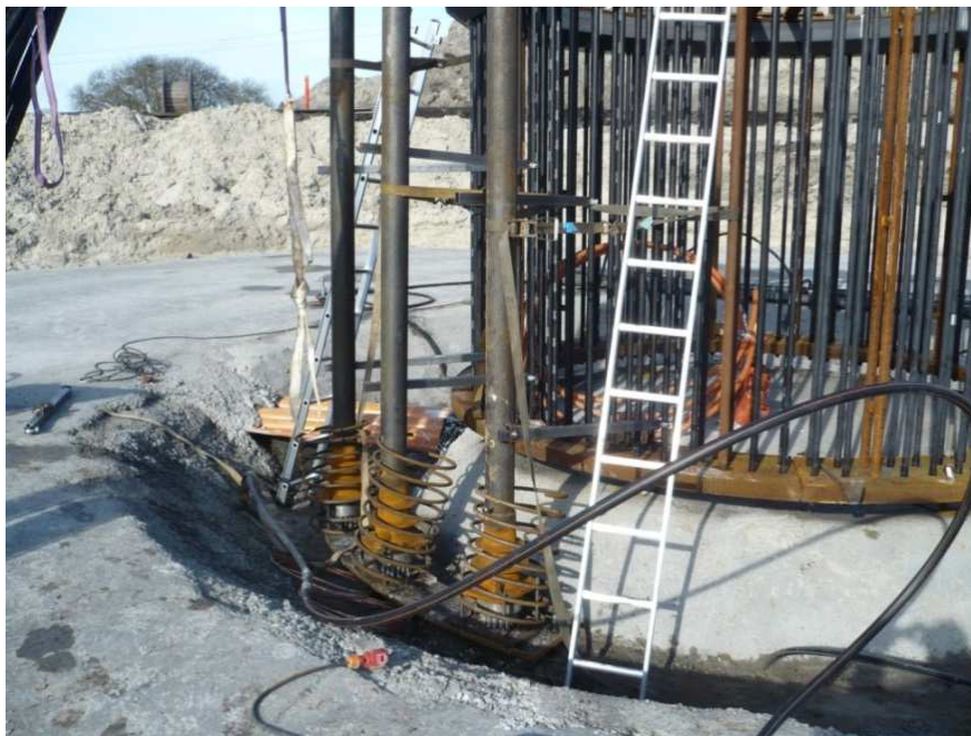
Foundation with both anchor bolts for a steel tower and post tension cables for a UHPFRC Hybrid tower
