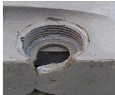
Figure 16. 4Defect around thread
