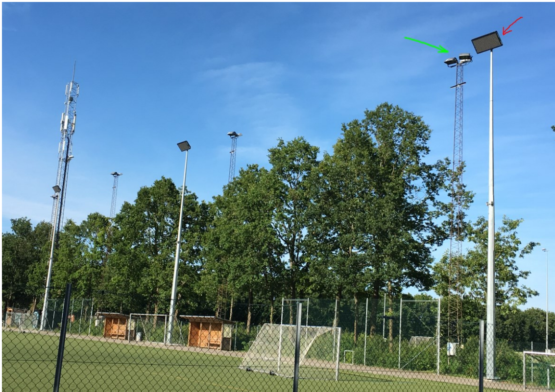
The Light installation at Himmelev/Veddelev Boldklub. The red arrow shows the new lamps mounted on new foldable 18m masts. The green arrow shows the old metal halide installation.
