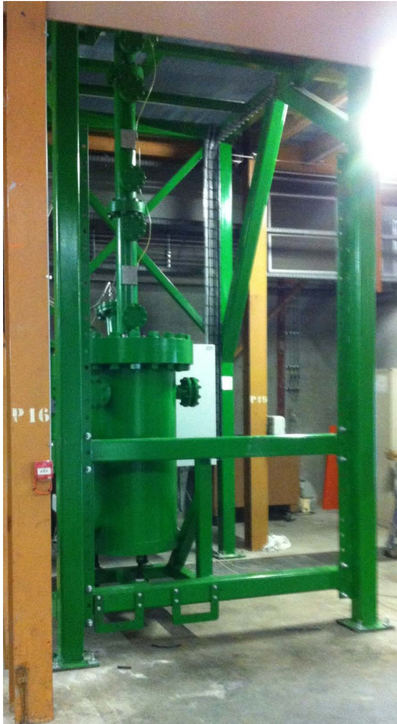
Figure 71 Picture of the ground floor of the facility with the receiver bin
