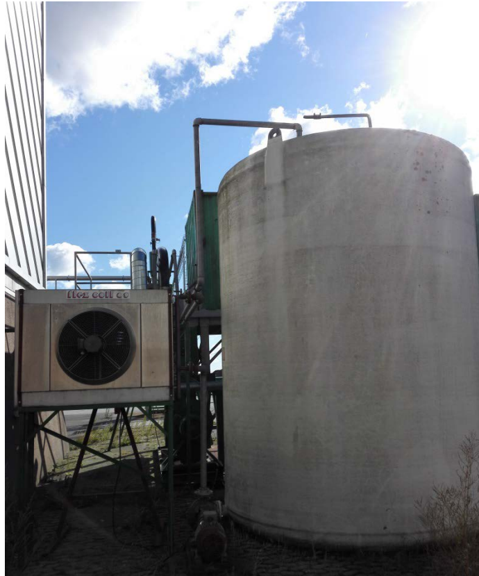
Figure 68 Picture of the water storage, pump and cooler
