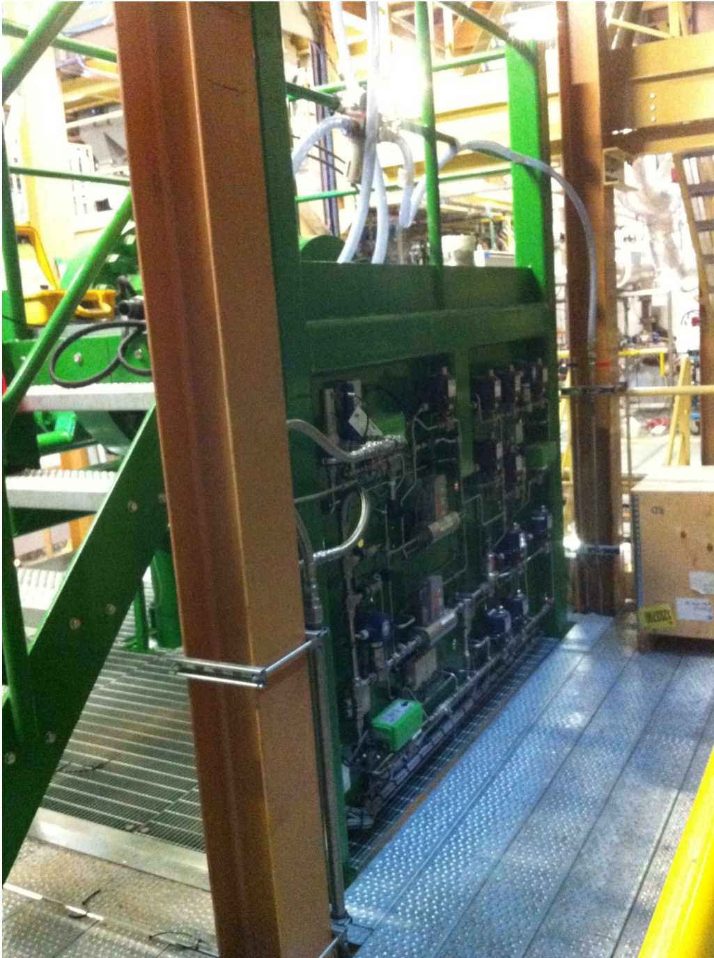
Figure 72 Picture of the gas system
