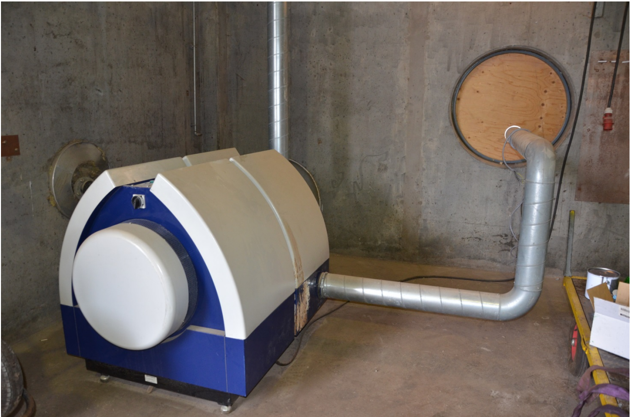
Figure 24 Picture of the blower supplying air to the dryer
