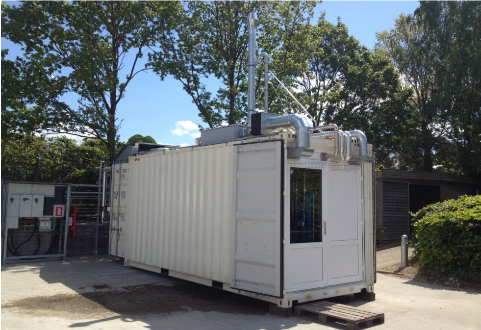
Figure 6.1 The eCOs plant utilising SOEC technology to produce up to 15 Nm 3 /h of on-site gas for the specialty gas market.
