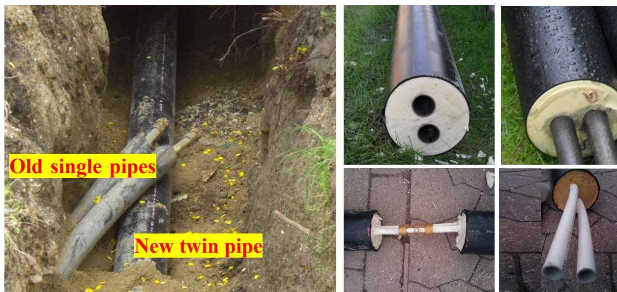
Figure A2.2: Example of a new twin pipe with good insulation property, which replaces the old single pipes with poor insulation thickness (to the left). Examples of steel twin pipes for the main network in the streets (upper right) and examples of alupex twin house-connection pipes – one of the pictures shows also a sampling before it is insulated and sealed with a casing (lower right). The pipes have inbuilt copper wires for leakage alarm system.
