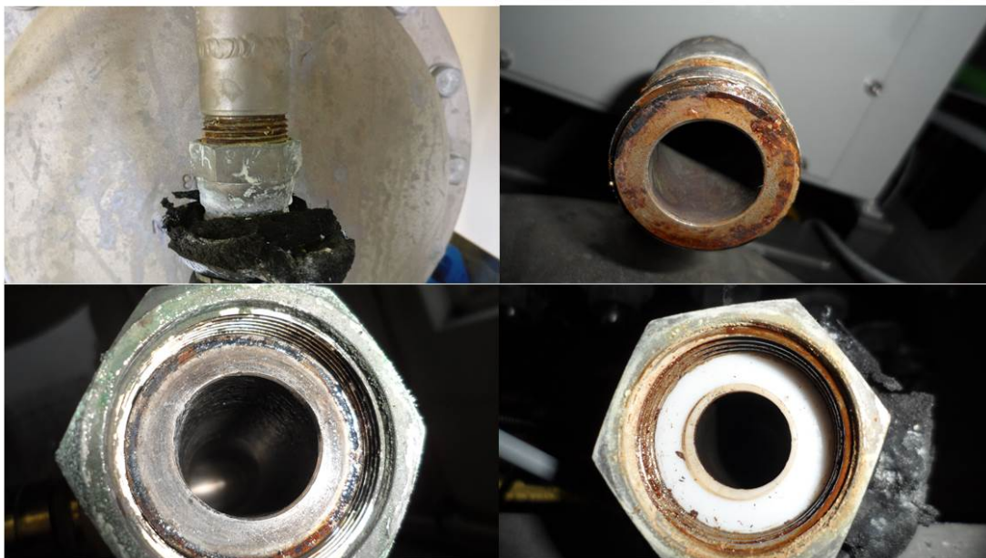
Figure 2 – Lye inlet at the separator. The connection is a Teflon Face seal with a 1”BSPP swivel. The separator and its connections are Ni-coated carbon steel. On the outside the regular surface shows no sign of corrosion, while the on the threaded part some surface rust is present, as the coating on the thread is very vulnerable, especially when the swivel nut is tightened. On the inside however, there are significant differences. On the hydrogen side (bottom left), the face still retains its shine, indicating the Ni coating for the most part is intact. For the Oxygen side (Top and bottom right), the sealing face have been damages and delamination of the coating have occurred. The inside of the fitting have similarly lost its lustre, indicating possible damage to coating. Regardless of the damage to the sealing face, the connection is still leak free.
