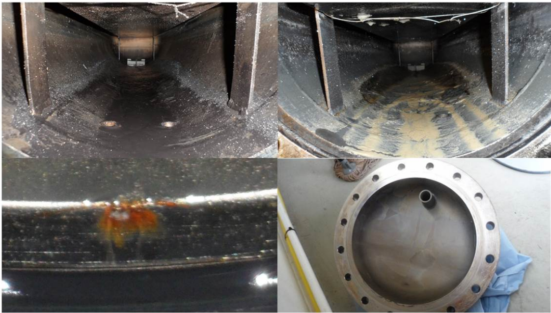
Figure 8 – Inside of the separators is seen some sludge in the bottom while the bulk of the coating it is intact. Some slight attacks are seen near the welds of the ramp brackets. There are also a few points where slight damage has been done to the edges of the flange because of mechanical chipping of the Ni coating on the edges. To prevent this, there need to be a chamfer on all sharp edges. The separators where the first parts to be manufactured with the electroless Ni-coating, so the experiences here have helped us design the parts to be better suited for the coating process.
