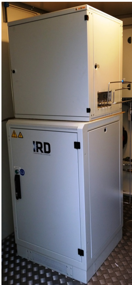
Figure 2: Electrolyser with dryer
