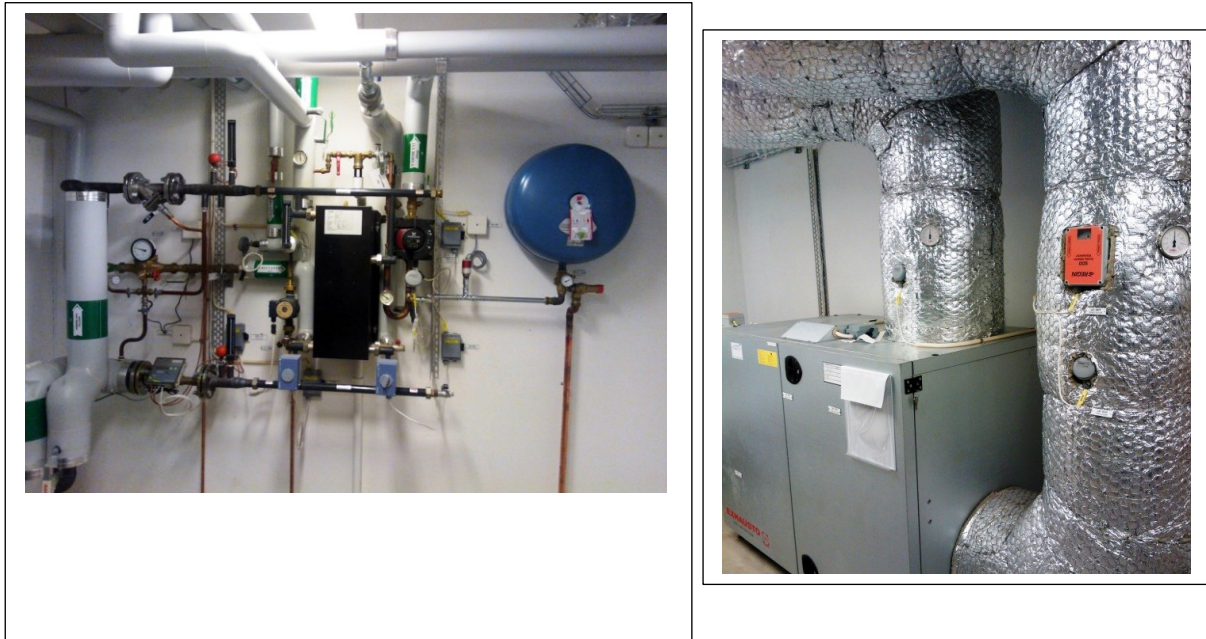
Figure 47. District heat plate heat exchanger sub-station installed at building ground level (left), and installation for exhaust air heat recovery to inlet air (right). Photos: The Author.
