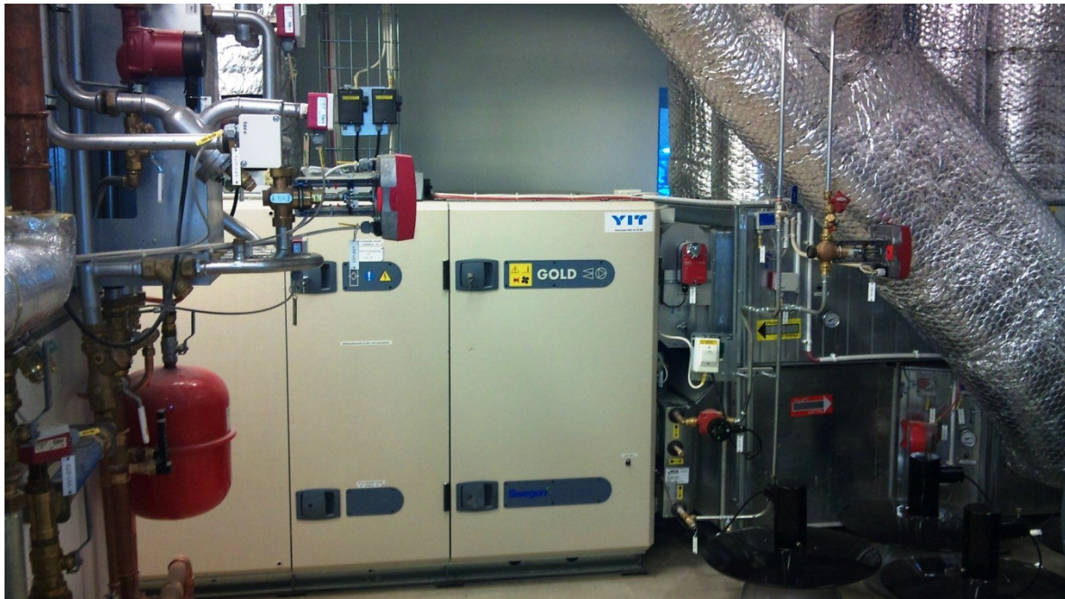
Figure 61. Forced air ventilation system with centrally placed rotating heat exchanger and subsequent district heat added as base load heat supply. Photo: The Author.
