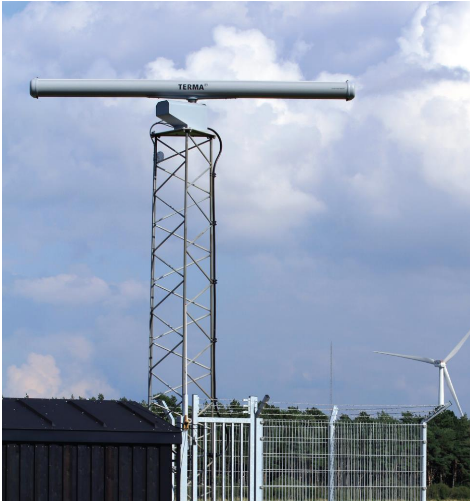
Figure 8 Radar OLC site in Østerild
