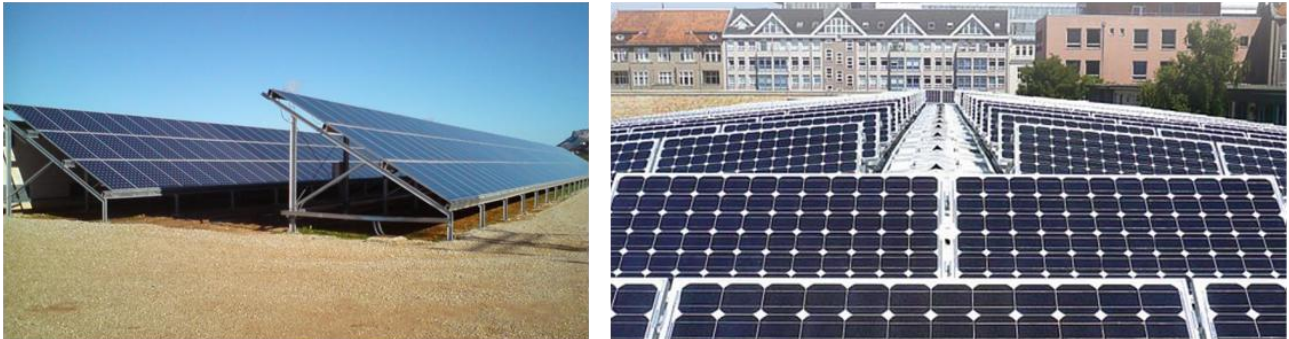
Figure 22: Ground mounted (left) and roof mounted (right) LPV installations.
