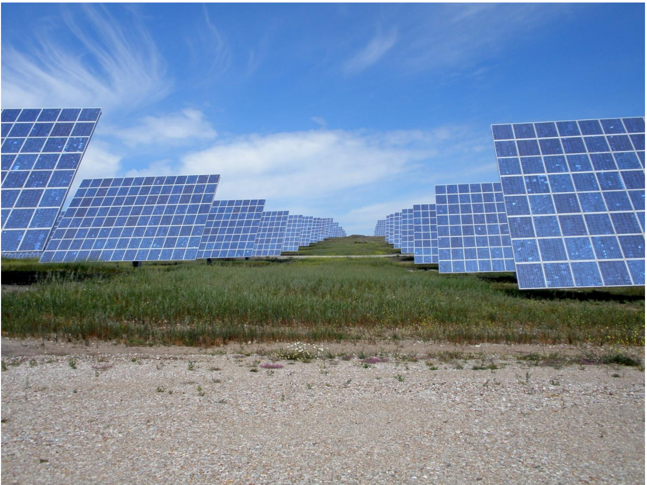
54 MW PV Plant in Moura Portugal; Photo: PA Energy Ltd.
