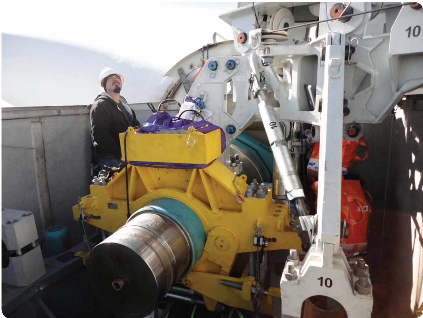
Main Shaft Fixture and Crane Base.
