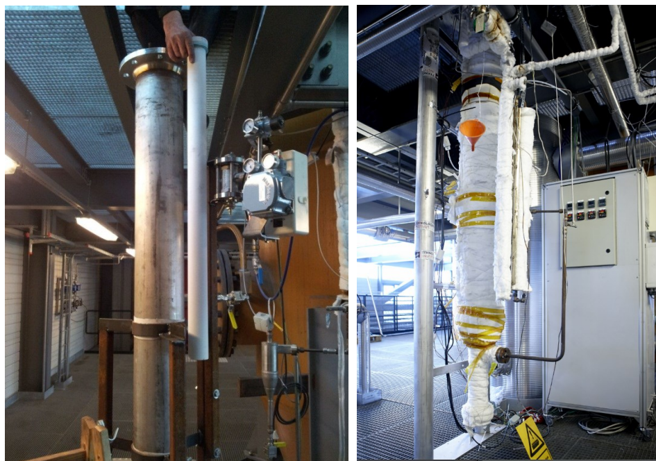
Figure 5: Filter element and filter house (left) and bottom of the reformer. Both photos are from the field test facility at Skive Fjernvarme
