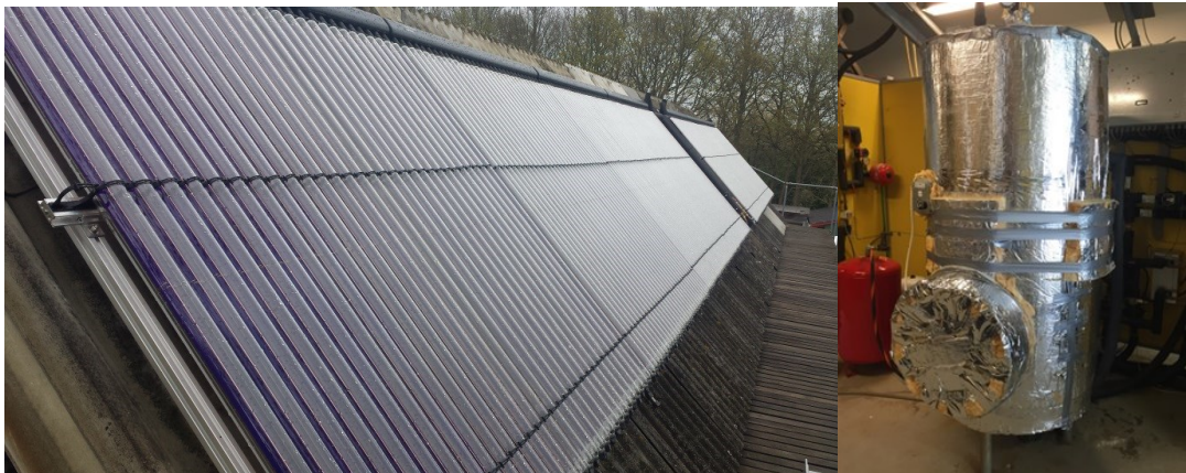
Figure 27. (a) Evacuated solar collectors for demonstration system. (b) 735 L water buffer storage for demonstration system.
